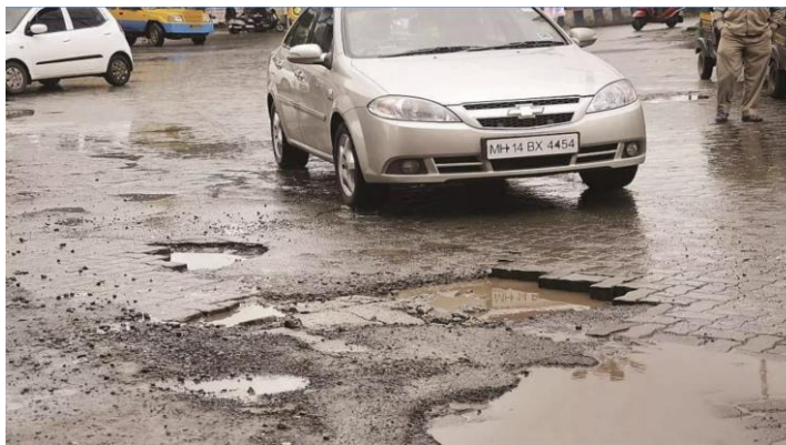
Poor Road Conditions
